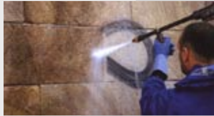
Sand stone protected by Fluoromer graffiti proofer. Graffiti can easily be removed.
